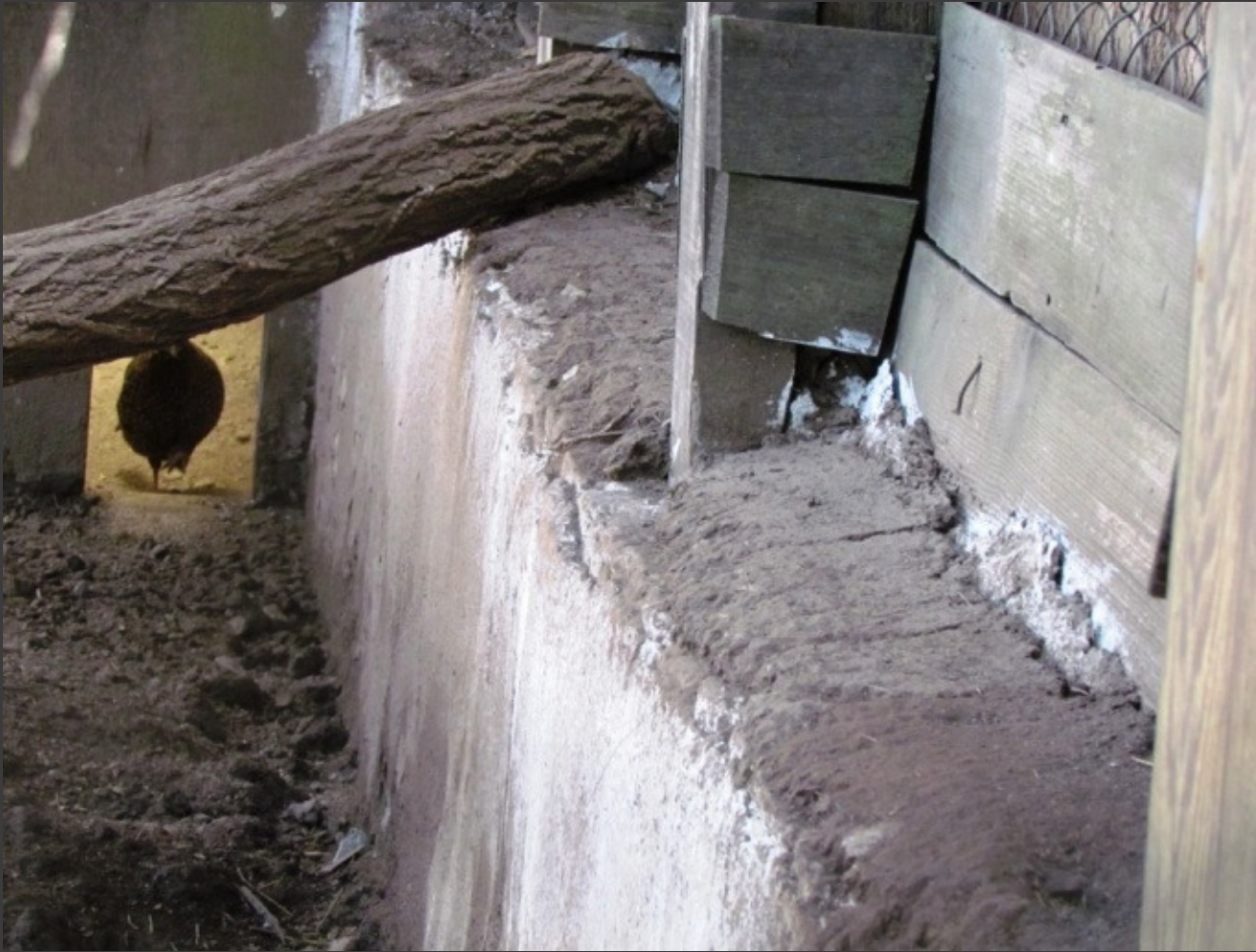
MUD PLASTERED CONCRETE SURFACES
